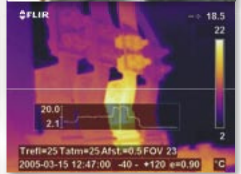
Top of transformer; low-voltage connection
