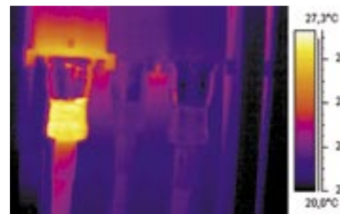
To decide whether a hot-spot is a real problem or not, you need to be acquainted with the installation.
