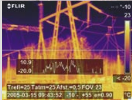
150 KV station, visual and thermal images
